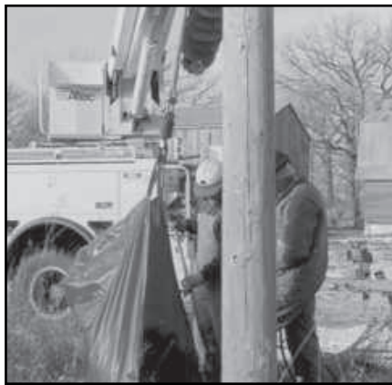
Winch dirt out of weeds. Trucks help put dirt back in hole. Tarp does not hinder tamping.
