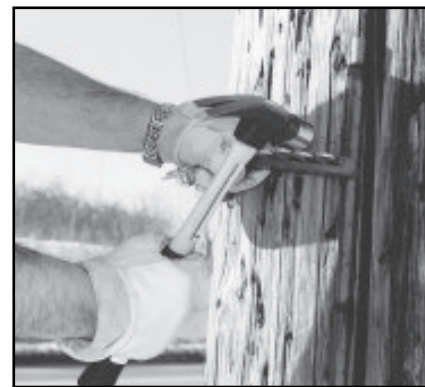
Hold the stick with staple over the ground wire, hammer top of staple to get started, pull staple stick away and set staple.
